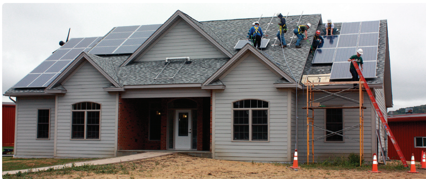
Students help to install solar panels atop Alfred State's net-zero model home.
