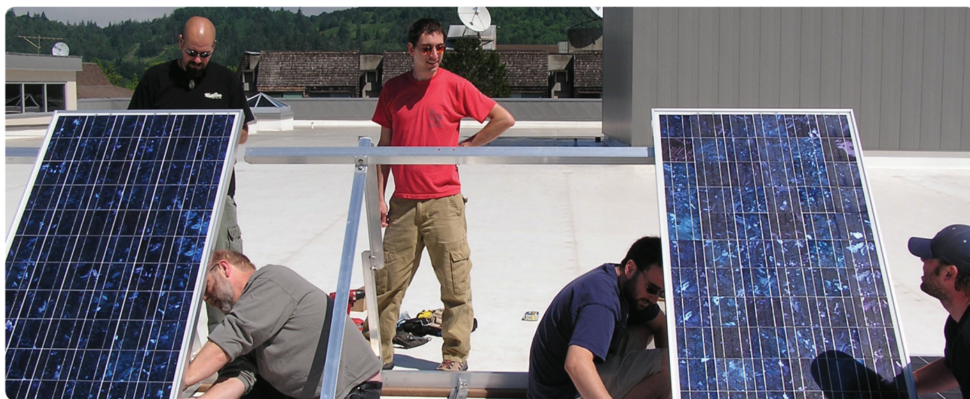
Students install a 1 kW solar PV system on the Lane Community College science building roof.
